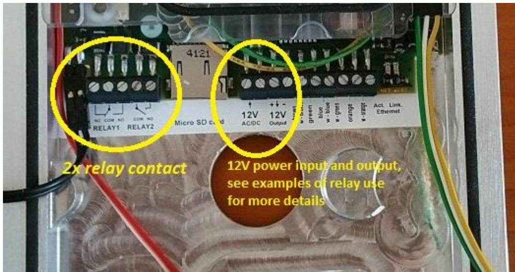
Fig 16 Terminal connectors for relays and 12 power input and output
